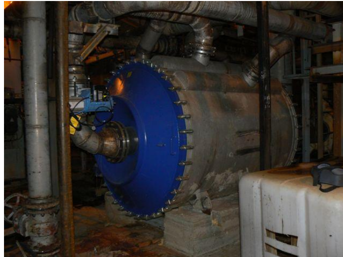
Fig. A.4-5. Spiral heat exchanger installed in the Cooking-and-Washing Department
